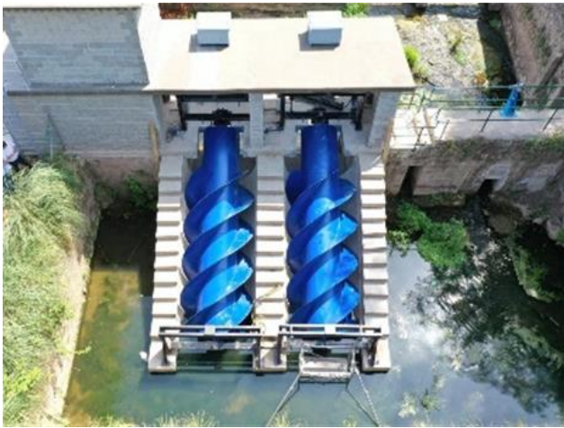
Fig. 6: Archimedes turbine at an industrial plant [7].
