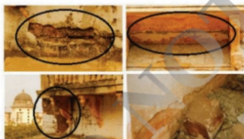
Figure 2. Major cracks and material deterioration of SH building.
