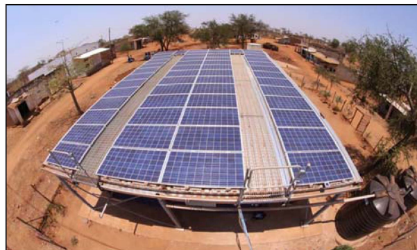
Figure 1: Bird's eye view of the 13.5 kW PV system in Makueni County, Kenya
