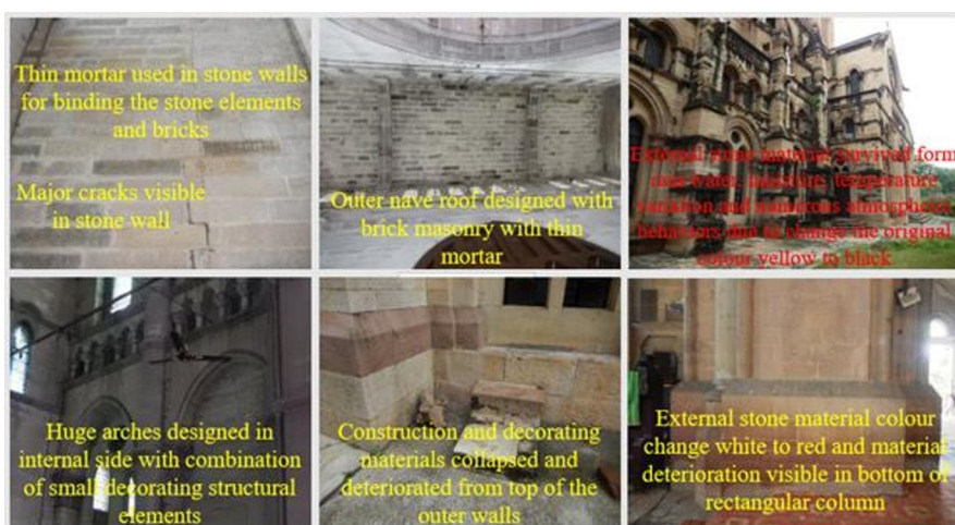
Fig. 11 Cracks and material deterioration of All saint cathedral church
