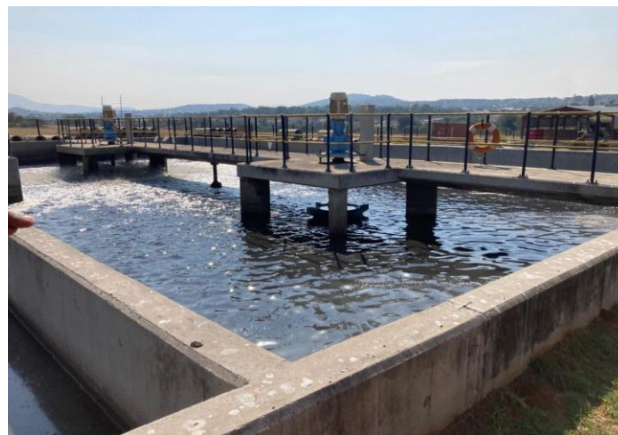
Fig. 5. Activated sludge wastewater treatment plant in South Africa (picture taken by the author)
